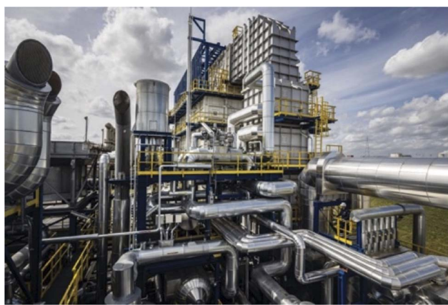
Fig. 14 One of the recent SMR-based H 2 production facilities (Air Liquide's SMR-X process) in Antwerp, Belgium, produces 99.99% pure H 2 at a rate of 56000 N m 3 per hour. The plant went into operation in April 2021. This shows the complexity of the plant and the stainless steel structures required in the form of pipes which carry hot gases.
