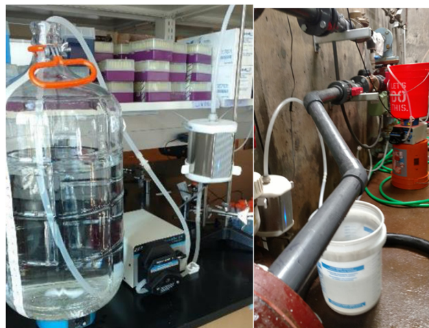
Fig. 35 UV LED reactor disinfection performance was assessed under varying conditions at bench scale (left) to develop a predictive model that was used to assess performance during challenge testing after pilot installation (right).
