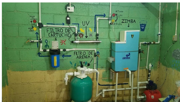
Fig. 5 Potable water treatment system installed in Escuela Primaria Aureliano El Mamey.
