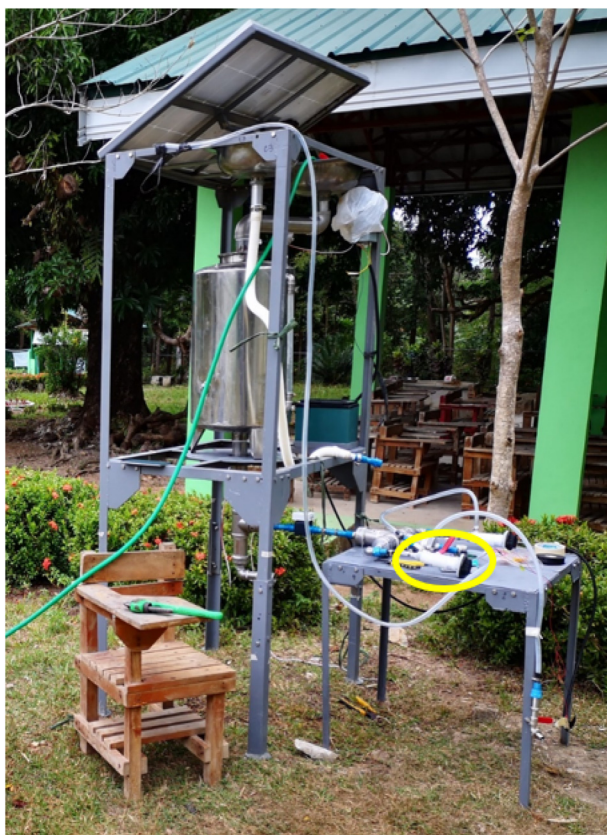
Fig. 22 Pilot setup of solar-powered UV LED water disinfection system in Panobolon Island, Guimaras, Philippines. The UV LED module is enclosed in the yellow circle.
