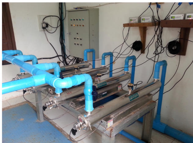
Fig. 15 UV disinfection system.
