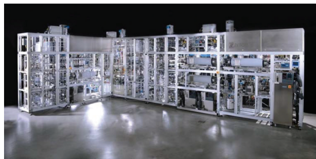
Fig. 2 Continuous API Manufacturing Pilot Plant supplied by Zeton to GSK. 36
