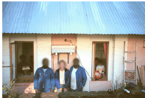
Fig. 29 UV Waterworks 2.0 unit installed on the exterior wall of the kitchen at the Lily of the Valley HIV-Hospice near Durban, South Africa.
