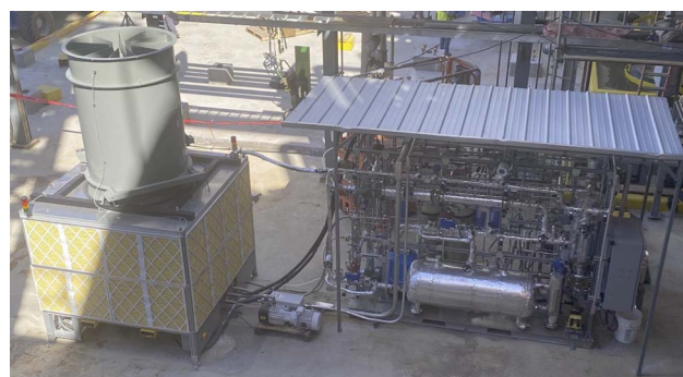
Fig. 5 One of Aircapture's DAC units (left) and collection skid (right). Located in Wilsonville, Alabama, USA at the US National Carbon Capture Center, this unit has been operating since March 2023.
