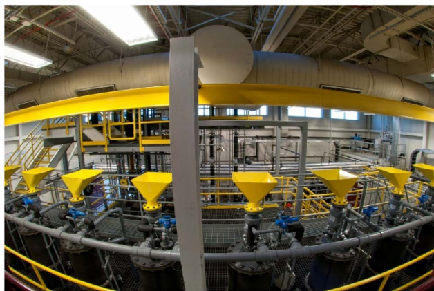
Fig. 18 Top side of the hydrolysis reactors at the Virdia pilot plant in Danville, the yellow conical funnels feed the wood material into the digesters.
