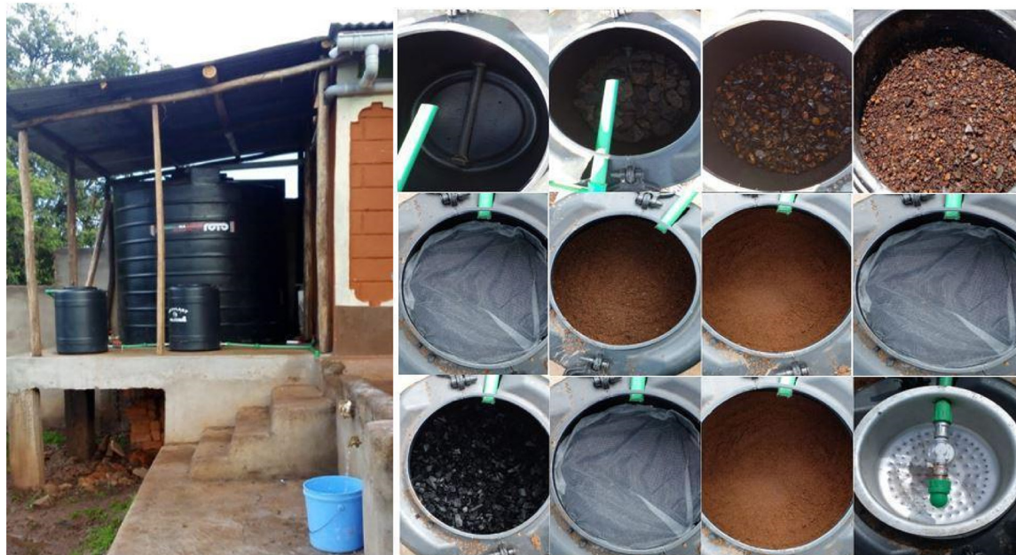
Fig. 17 (Left) Rainwater collection, filtration and disinfection system. (Right) Biosand and biochar layers within the filtration system.
