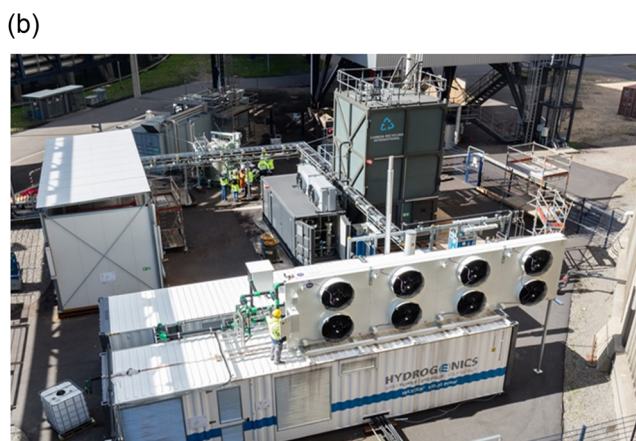
Fig. 19 (a) Schematic of the MefCO 2 plant 77 and (b) the actual pilot-scale MefCO 2 plant (right) at RWE's lignite-fired coal power plant in Niederaussem, Germany. 104
