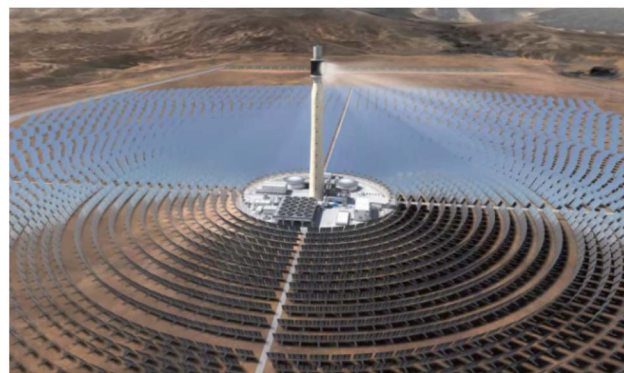
Fig. 6 Aerial view of the Ouarzazate Solar Power Station in Morocco. Image adapted from cited ref. 76.
