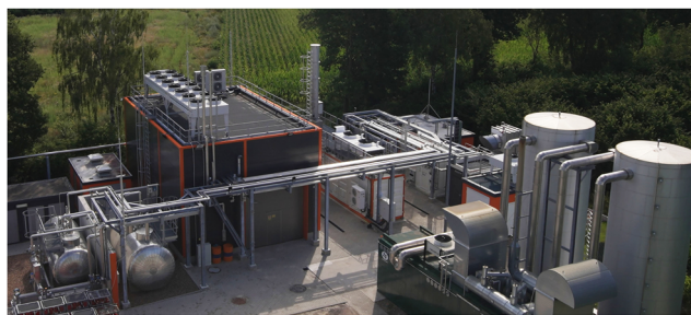
Fig. 24 Actual site of the 350 tpa of SAF production plant at Werlte in Germany, including the electrolysis system that forms the core of the plant. 114,115
