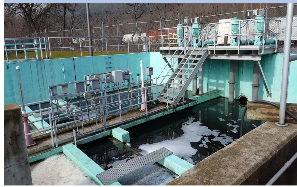
Municipal Wastewater Treatment Plant
