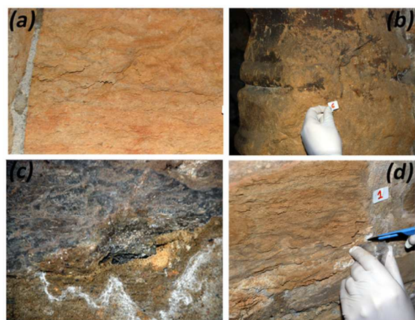
Fig. 2 Photographs of the deterioration observed in the Palace House; (a) Details of flaking over sandstone of the central courtyard, (b) Sandstone structural column details of the central courtyard, (c) Enlargement of the salts front with an important material loss, in the first instance, (d) Details of efflorescences and subefflorescences over sandstone of the central courtyard.
