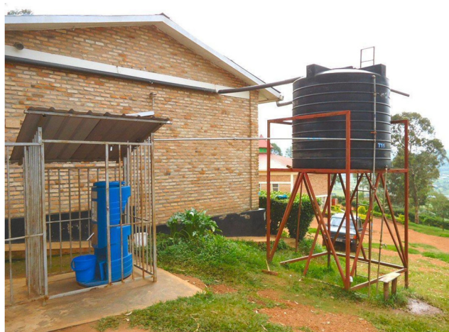
Fig. 25 A Naiade (on the left) and rainwater harvesting tank on a primary school in Kigali, serving 240 children and 20 staff members.
