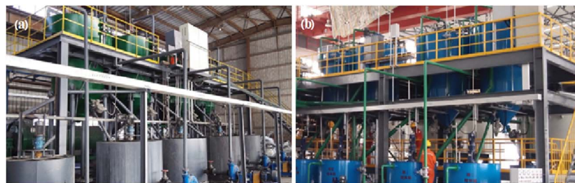
Fig. 8 Carbon dross flotation production line. (a) A 6 kt a -1 treatment line in Henan, China and (b) a 20 kt a -1 treatment line in Liaoning, China.
