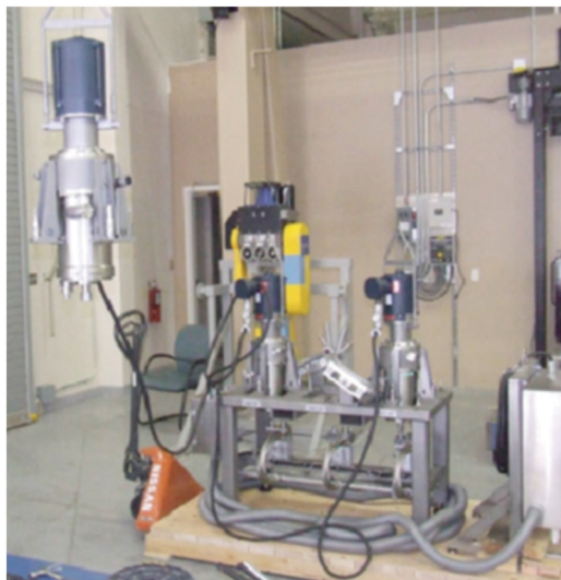
Fig. 35 Centre position V-05R contactor unit removed from a cascade of 3 stages of 127 mm RD CCs in a simulated highly radioactive environment.
