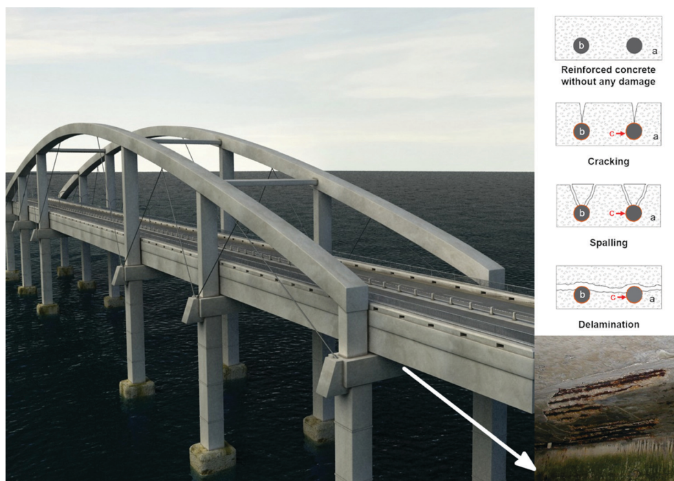
Fig. 3 Bridge with a schematic representation of cracking, spalling or delamination in a RCS where “a” represents the concrete, “b” the rebar and “c” the oxide layer. The photograph in the bottom right corner shows the typical feature of concrete detachment due to rebar corrosion.
