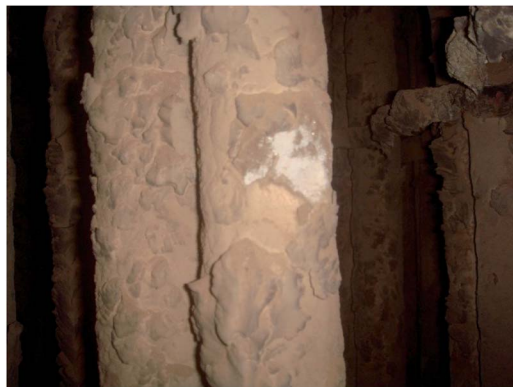
Fig. 2 Deposits on high temperature superheater.
