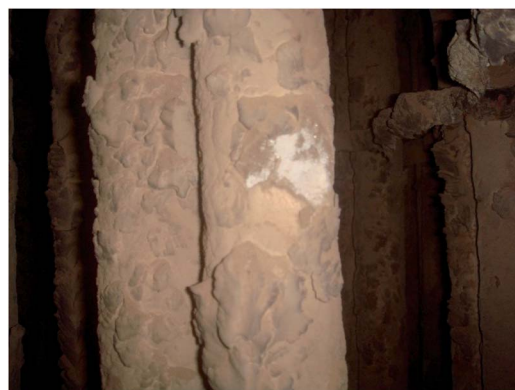
Fig. 2 Deposits on high temperature superheater.
