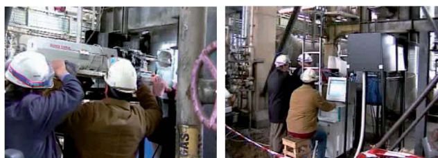
Fig. 6 LIBSGRAIN project: mounting of the laser at the plant for pipe analysis (left) and mapping of steel composition (right).
