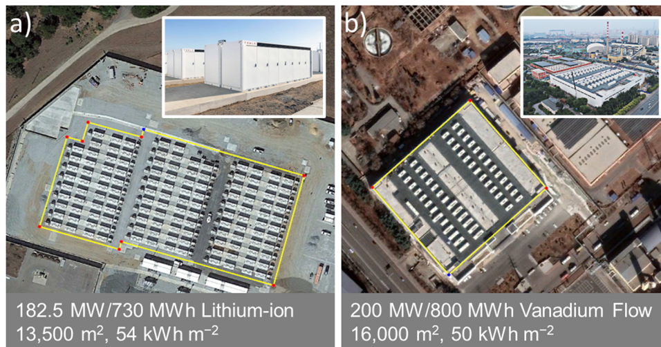
Fig. 2 Satellite images and photos of some of the largest battery energy storage systems deployed to date. (a) Lithium-ion batteries in Moss Landing, California: Elkhorn Battery, operated by Pacific Gas & Electric Company; 182.5 MW/730 MWh, 54 kWh m -2 . Map Data: Google, © 2022 AMBAG, Maxar Technologies, Photo adapted from ref. 42. (b) Vanadium flow battery in Dalian, China, by Dalian Rongke Power Co. Ltd; 100 MW/400 MWh, 25 kWh m -2 . A second phase of equal capacity in the same building is under construction, bringing the areal energy density to 50 kWh m -2 . Map Data: Google, © 2022 Maxar Technologies, Photo adapted from ref. 43.
