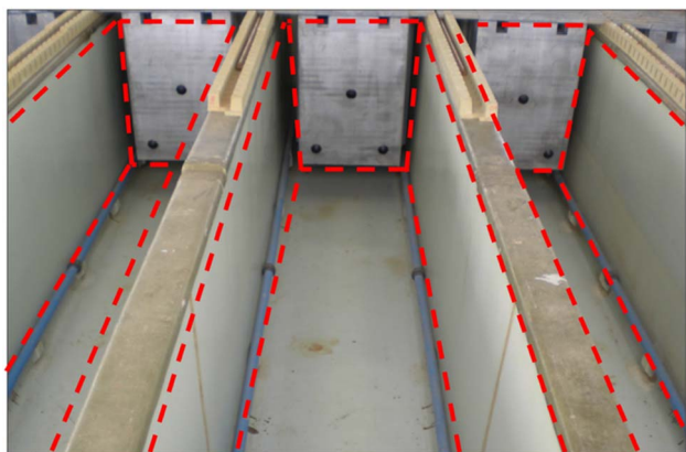
Fig. 10 Industrial scale setup of copper electrowinning. The implementation of such a setup could be a 'blueprint' for feasible large-scale setup of the electrochemical recycling process.
