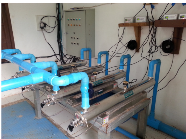
Fig. 15 UV disinfection system.
