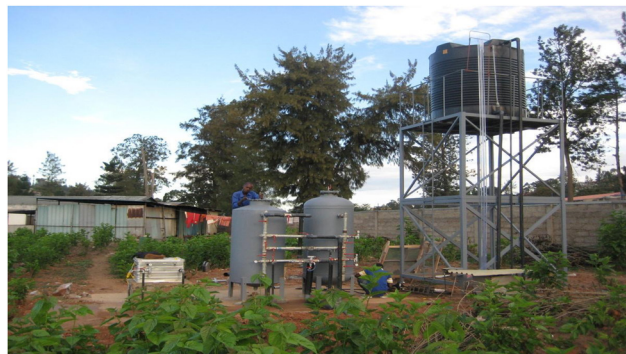
Fig. 27 An example of the Manna Energy Limited water treatment system. The system is installed in-line with existing water pipes. On the right is an elevated backwash tank. In the center is a gravel filter and a pressurized sand filter. On the left is the solar photovoltaic-powered UV system.
