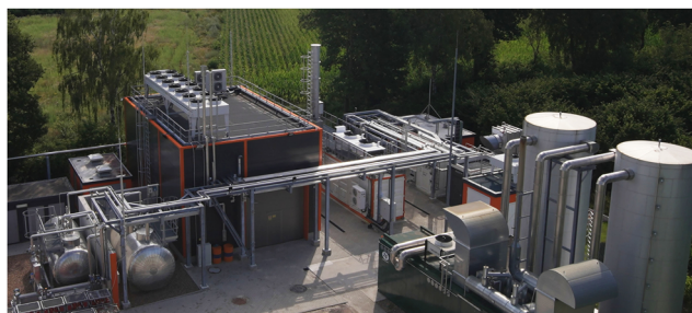
Fig. 24 Actual site of the 350 tpa of SAF production plant at Werlte in Germany, including the electrolysis system that forms the core of the plant. 114,115
