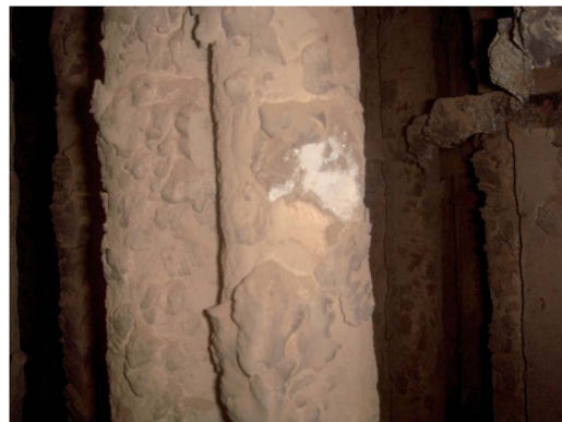
Fig. 2 Deposits on high temperature superheater.
